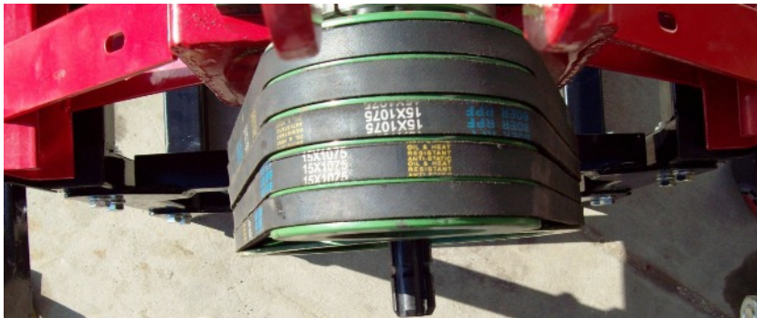
Bad Horizontal Alignment
